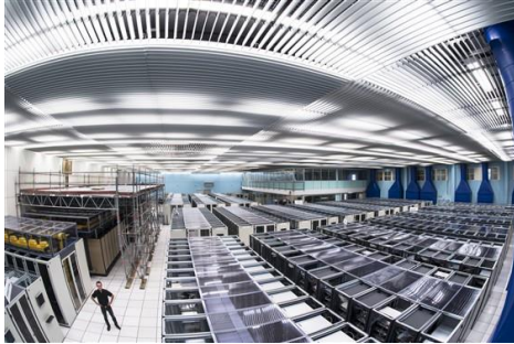
CERN Data Centre [6]
